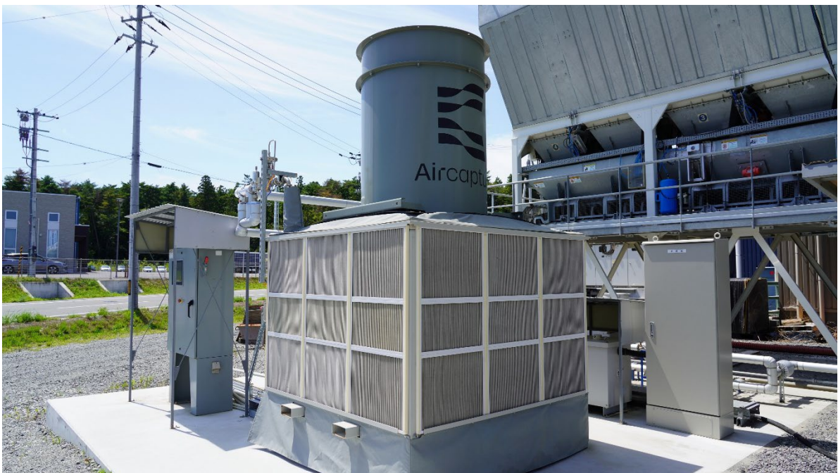
a DAC system installed at AIZAWA Concrete's Fukushima RDM Center
