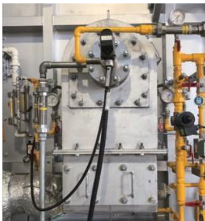
Regenerative burner exterior
